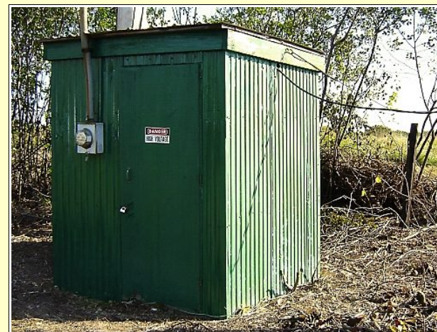
This building is about 50 feet from the telephone building. It was originally used by the power company for their two-way radios on low band. Two 45 foot cedar poles are next to the building and are also in good shape. An underground power line was installed between the buildings by the Ham club so one electric meter serves both.
