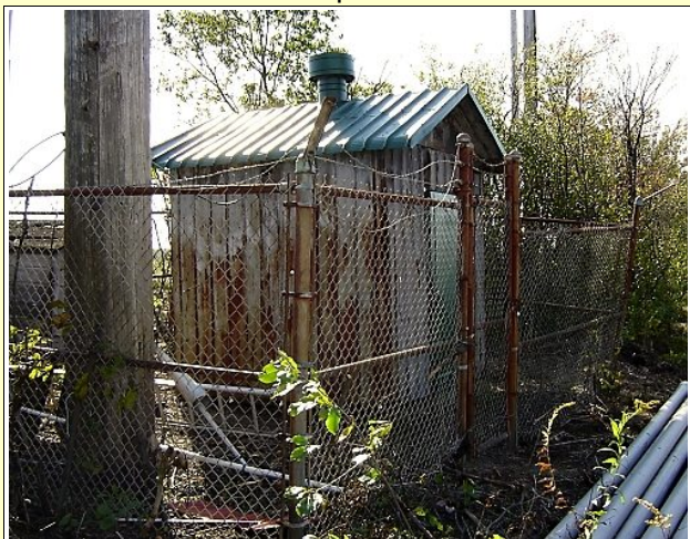
The original Home Telephone Company radio building from the '60s. Amazingly, the roof and metal skin are in good shape. The skirt of the building did show some rust but was sealed with expanded foam. The 70 foot cedar pole is next to the building inside the fence.
