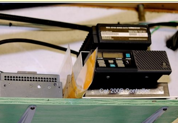
Dutch Hill Receiver installation (Potter County)
