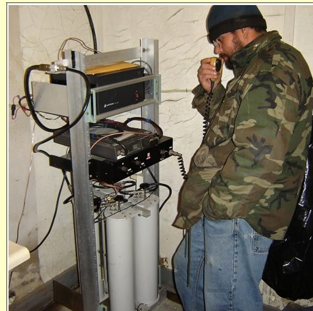
Joe N3UGB makes the first contact on the 147.00 MHz repeater from the new radio site. A Poly-phaser lightning arrestor is installed on the left upper rack support and grounded with #6 copper ground wire to a very extensive grounding field outside the building.
